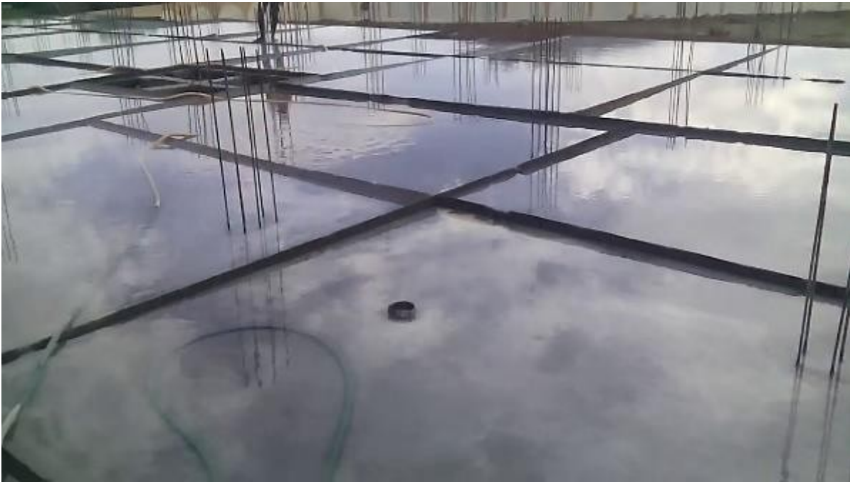
Fig.: Ponding of concrete
