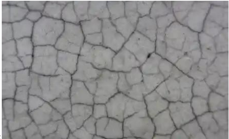
Fig 2: Crazing or Pattern Cracking
